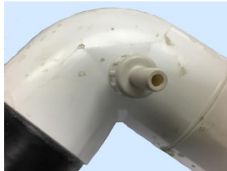
Figure (6) AABV Installed in Rigid PVC Elbow
